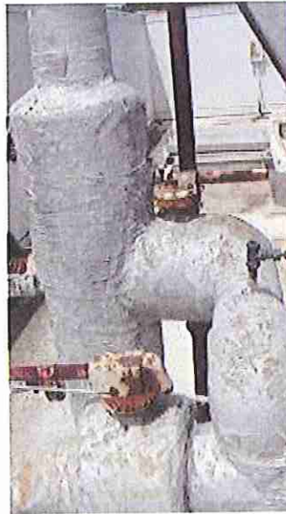
Figure M22: AHU's isolation valves showed extensive corrosion
