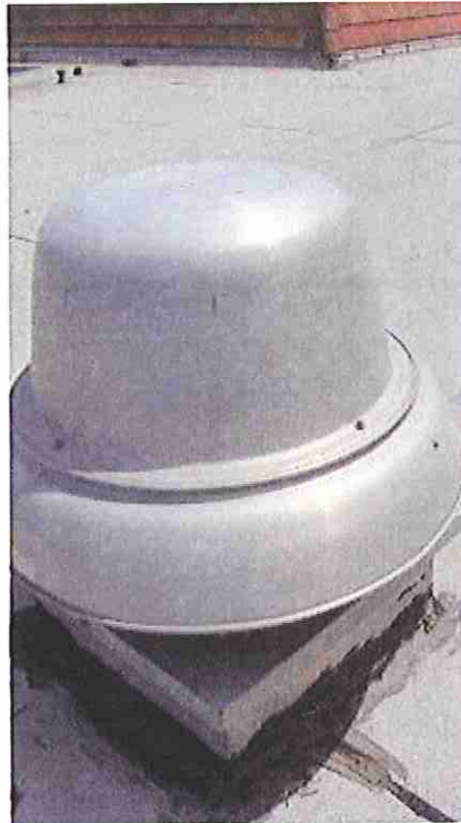
Figure M15: E-8 Exhaust Fan
