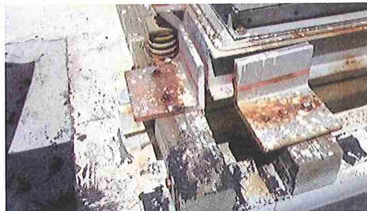
Figure M3: AHU's Isolator & Snubbers
