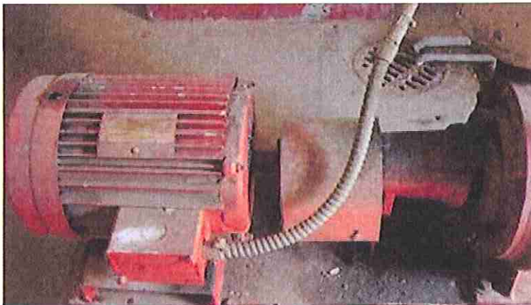
Figure M17: Chilled Water Pump
