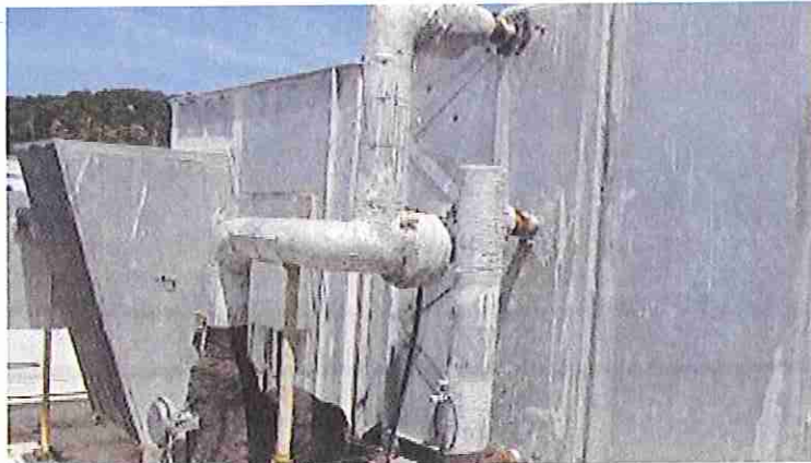
Figure M1: AHU-1 Right Side
