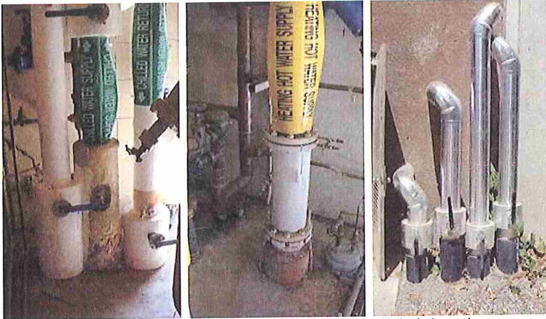
Figure M19: Chilled & Heating Water Risers with isolation valves.
