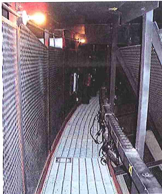
Figure 12 – Theatrical Lighting along the Catwalk
