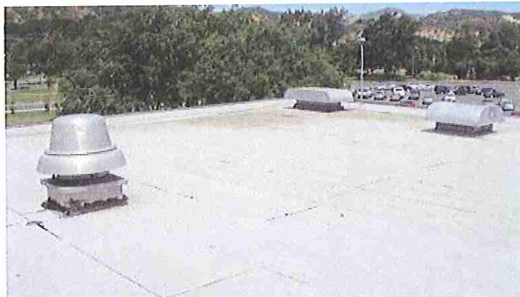
Figure M13: E-5 & E-6 Exhaust Fan
