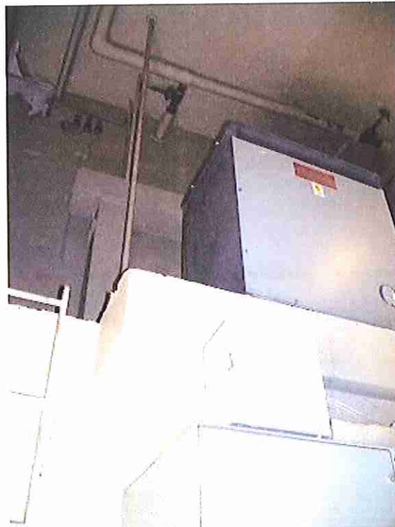
Figure 3 – Plumbing Water Pipes above the Electrical equipment
