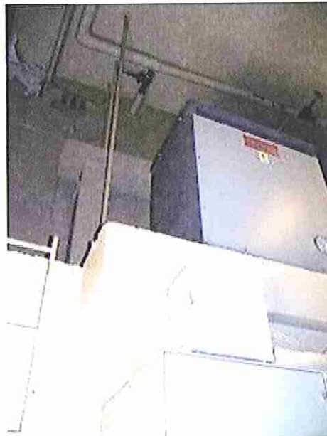
Figure P2: Domestic cold water isolation valves above electric transformer & equipment.
