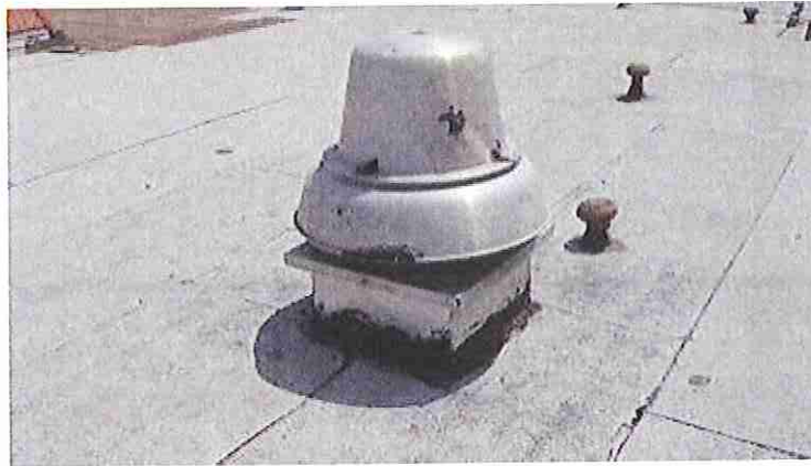
Figure M12: E-4 Exhaust Fan
