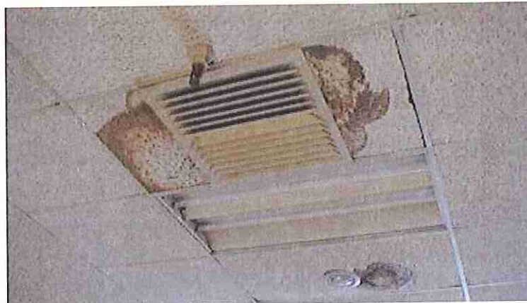
Figure M20: Air supply register at the ceiling.
