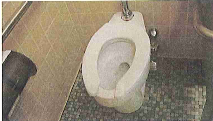
Figure P3: Toilet with flush valve
