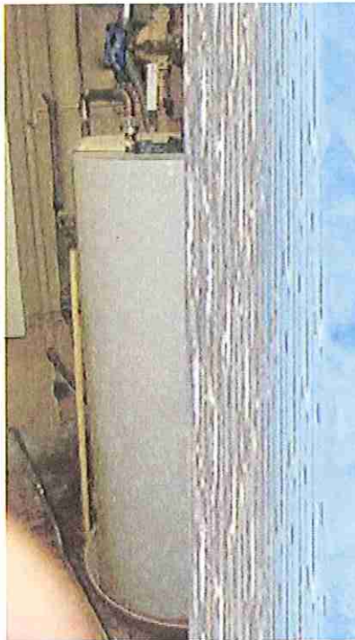
Figure P8: Electric water heater
