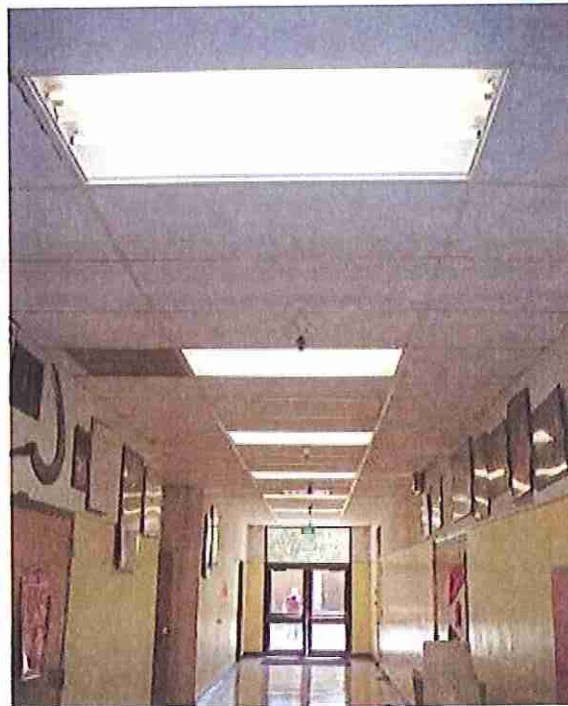
Figure 8 – Typical Corridor Lighting
