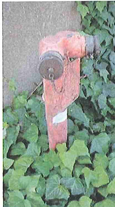
Figure F2: Fire Department Connection
