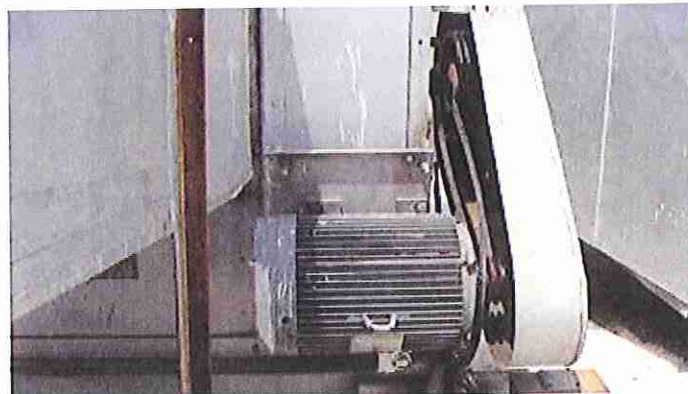
Figure M21: AHU-2 fan belt is snapped, motor is still running!
