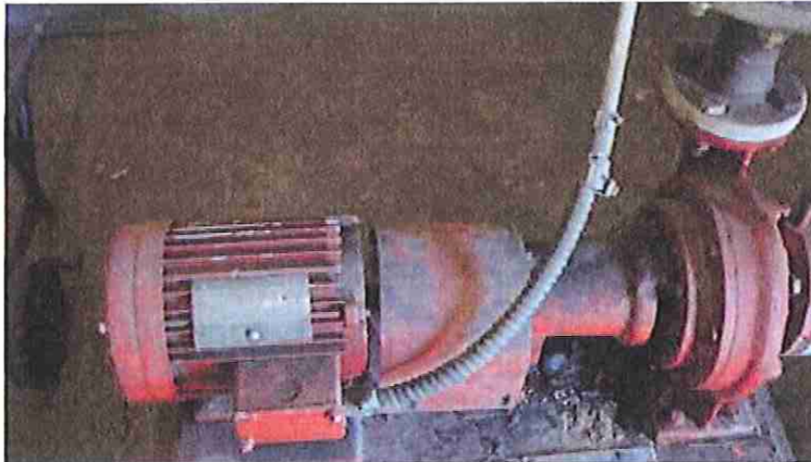
Figure M16: Heating Water Pump
