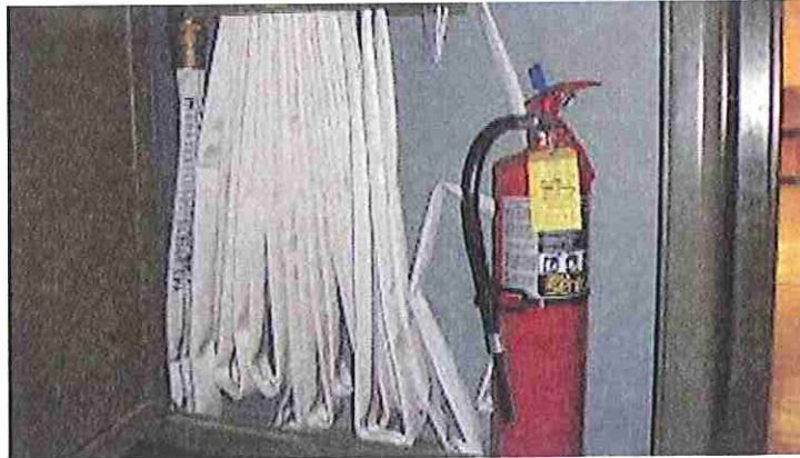
Figure F3: Fire Hose Cabinet
