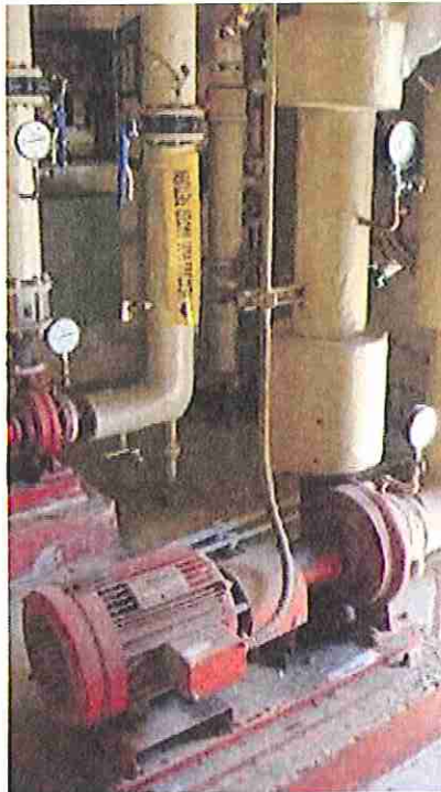
Figure F1: Fire Riser Tucked in Corner
