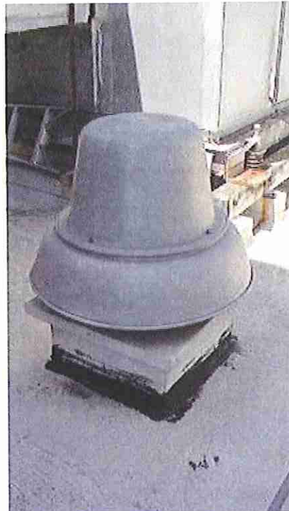
Figure M10: E-2 Exhaust Fan
