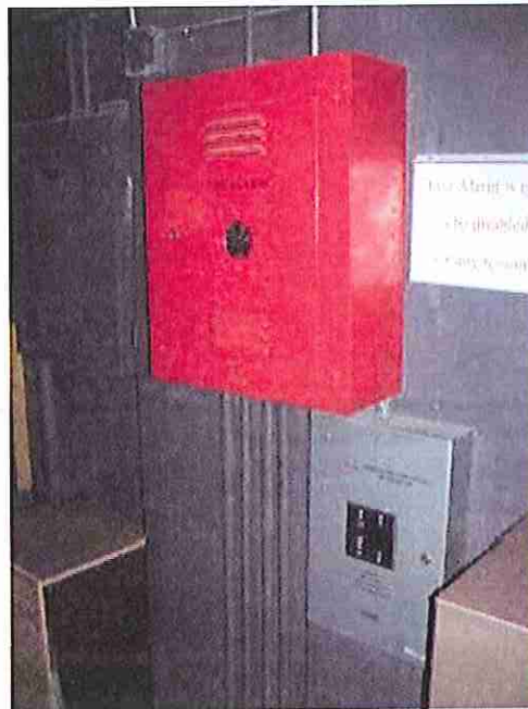
Figure 13 – Fire Alarm Control Panel behind the Stage in the Theater Area
