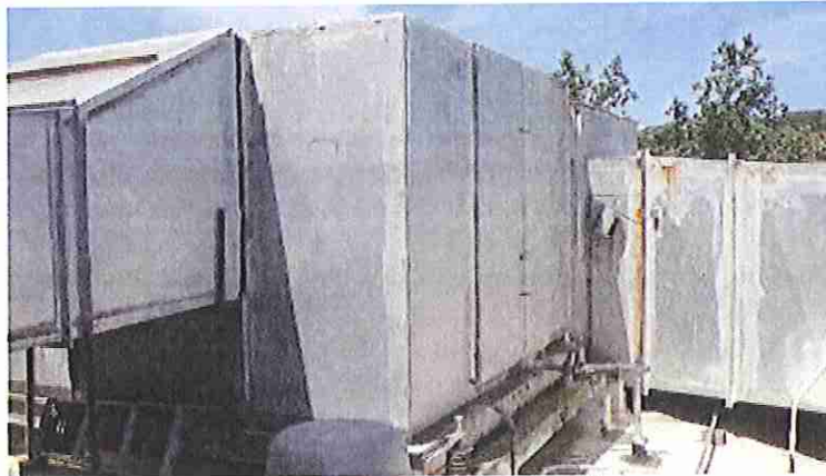
Figure M2: AHU-1 Left Side
