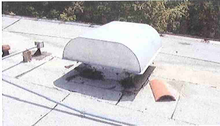
Figure M14: E-7 Exhaust Fan
