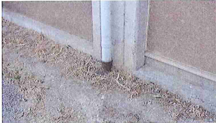
Figure P7: Typical rainwater leader hard-piped to site storm drain system.
