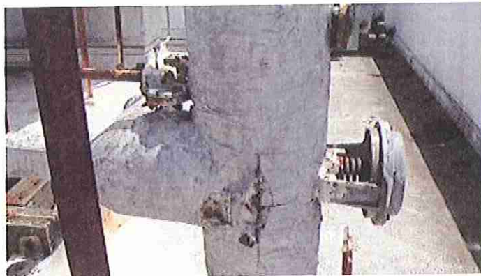
Figure M23: AHU's control valve showed extensive corrosion
