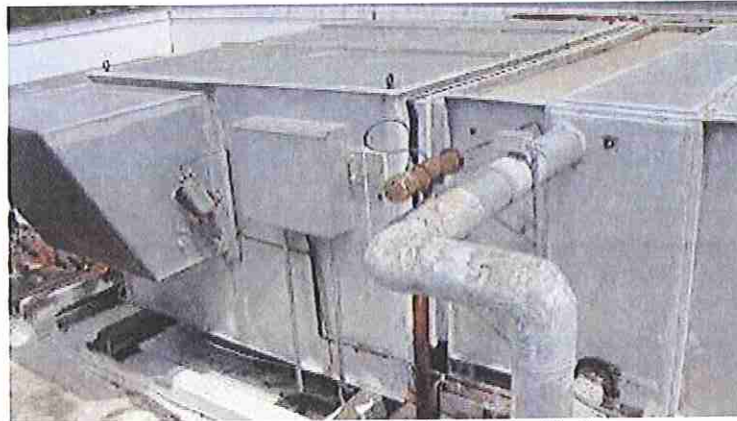
Figure M7: AHU-2 Air Handling Unit.
