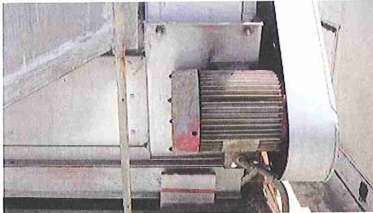
Figure M6: Return fan motor with bad bearing.
