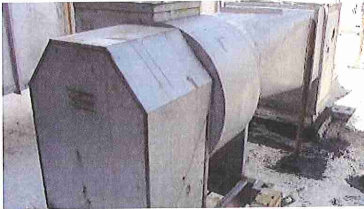
Figure M9: E-1 Exhaust Fan
