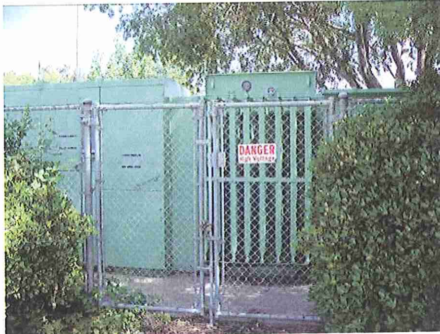
Figure 1 – Substation #1 located South of Building 1200
