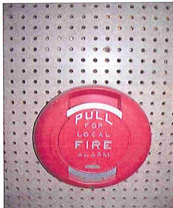
Figure 14 – Typical Fire Alarm Pull Station
