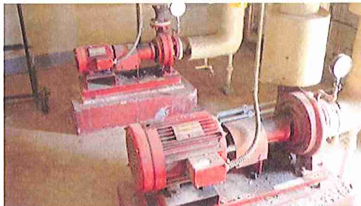
Figure M18: Heating & Chilled Water Pumps
