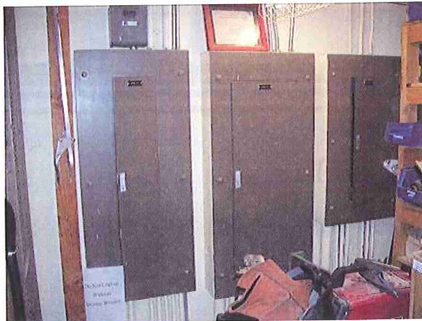
Figure 4 – Branch circuit panelboards in Shop Room
